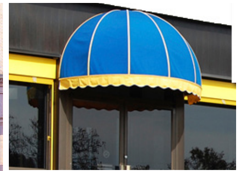
Example of Unacceptable Awning
